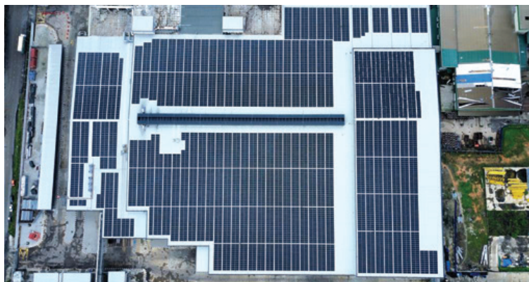
Solar Panel on the roof top of the primary processing plant
