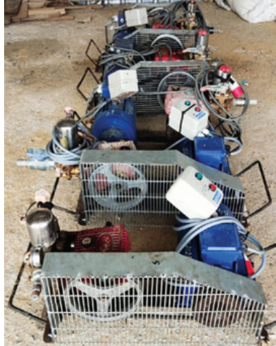
Safety Guarding for all Water Pump Rotating Belt at farm
