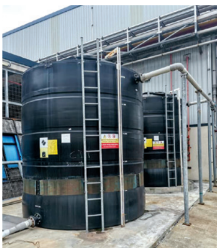
Harvested Rainwater Tank
